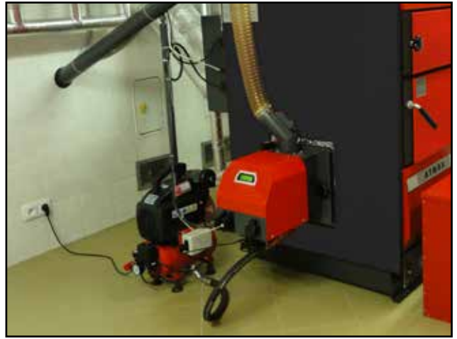
Compressor set up beside boiler
