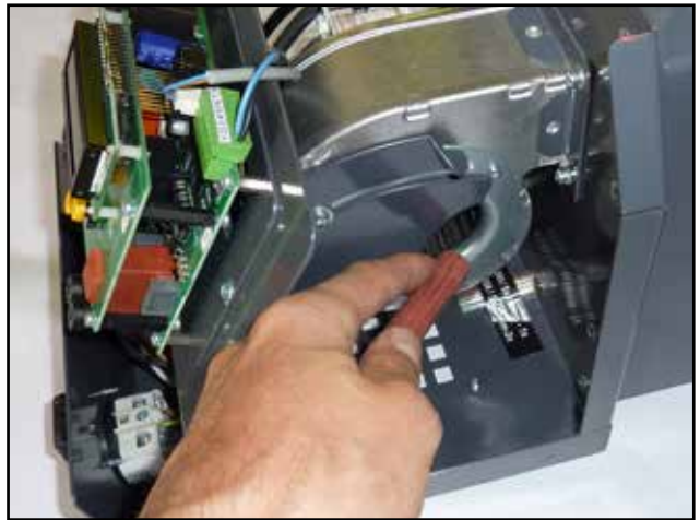
Example of cleaning (blow out) pressure fan impeller of the burner once a season
