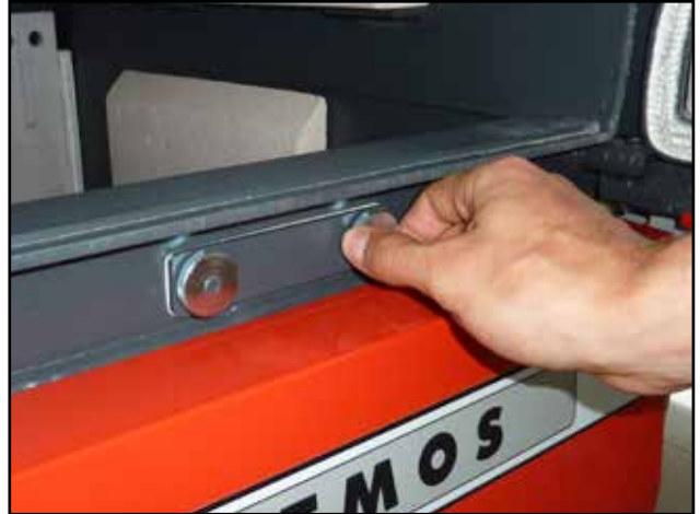
Tightened additional secondary air cap for DxxP, Pxx boiler
