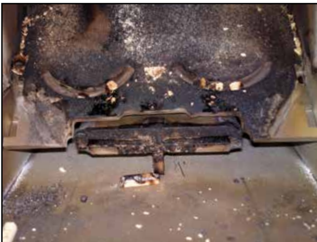
Slight clogging after 4 months of use
